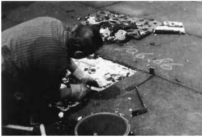
Fig. 1 Removing the roof covering to inspect Styropor foam panels that had been installed 31 years before. The joints between the panels were still tight.
