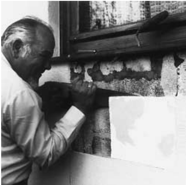
Fig. 3 Taking a sample of Styropor from an outdoor composite insulating system consisting of Styropor and a fabric-reinforced textured finish.
