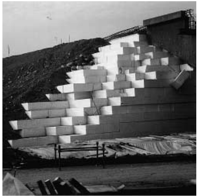
Fig. 7 Styropor blockware in the construction of causeways and bridge ramps in regions with poor load-bearing soils (European Highway E6, Ljungskile, Sweden).
