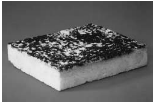
Fig. 2 Specimen taken from flat roof as shown in Fig. 1. No changes can be discerned in the Styropor.
